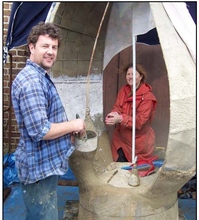
"Sea Harmony" mosaic sculpture construction underway at the Arts Company with Annette & Tony.
