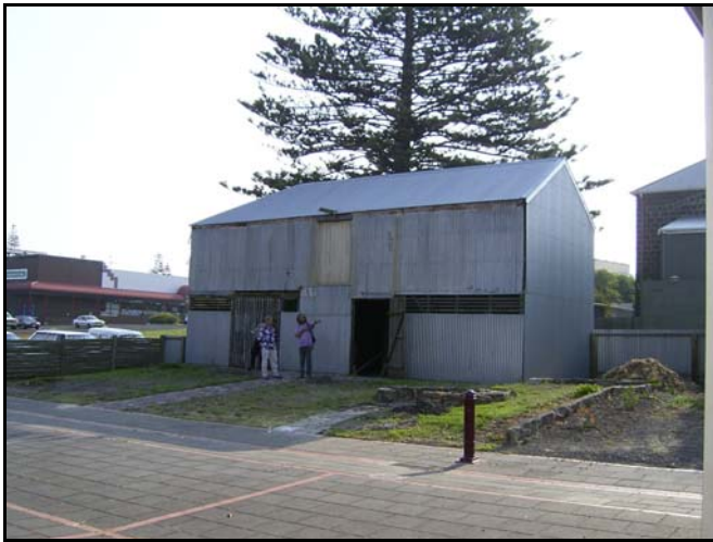
The Stables, recently the subject of a conservation project by Gordon Stokes, Workskills, and participants of the Work for the Dole Scheme
